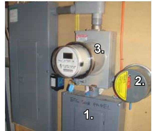
IN CONTROL: In this scenario, all electricity that flows through a subpanel (1.), attached to a main panel in a home, is priced at the controlled/interruptible rate. A load control switch (2.) controls power to the subpanel, which has its own meter and meter base (3.).
