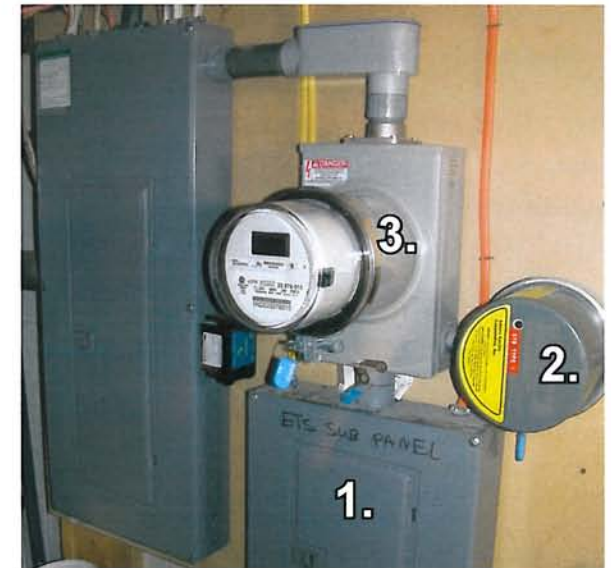
IN CONTROL: In this scenario, all electricity that flows through a subpanel (1.), attached to a main panel in a home, is priced at the interruptible rate. A load control switch (2.) controls power to the subpanel, which has its own meter and meter base (3.).
