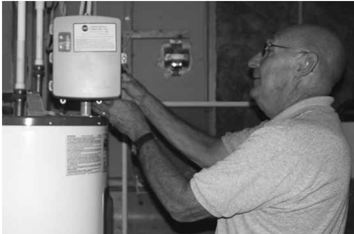
New load control switches on water heaters bring greater reliability for the load control program.
