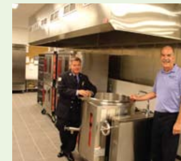
SAVES FIRE COMPANY WAS ABLE TO INSTALL A STATE-OF-THE-ART KITCHEN USING FUNDS FROM THE CO-OP'S CD FUND PROGRAM.
