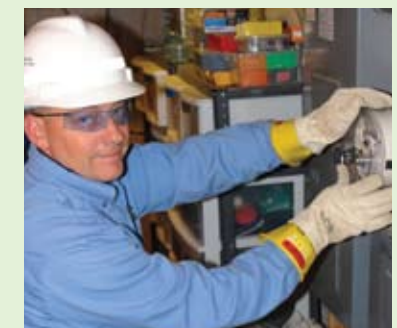
A SERVICE TECHNICIAN FOR ADAMS ELECTRIC INSTALLS A NEW CONTROLLED/INTERRUPTIBLE METER AT A MEMBER'S HOME. THE METER CONTROLS THE ELECTRICITY USE OF AN ETS HEATING UNIT, A WATER HEATER, A DRYER, A DEHUMIDIFIER AND A BACK-UP AIR-SOURCE HEAT PUMP, ALL PLACED ON THE CONTROLLED/INTERRUPTIBLE RATE.
